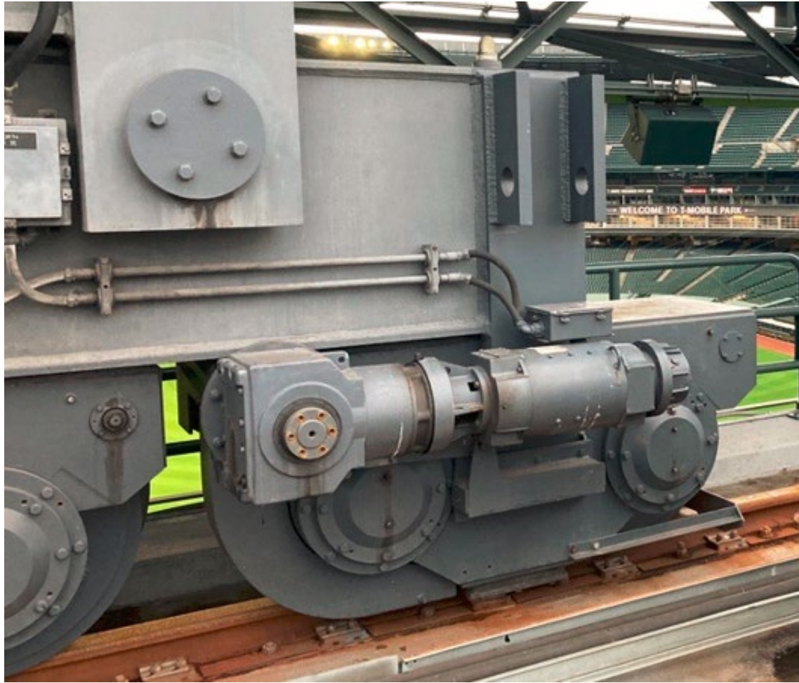
Figure 3: Retractable roof's wheel drive.
