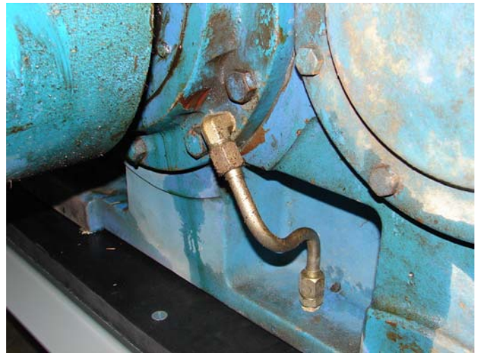
Figure 19. Low Speed Grease Relief Line
