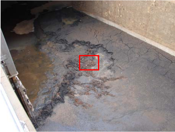
Figure 6. Aerator 1 Basin Sediment
