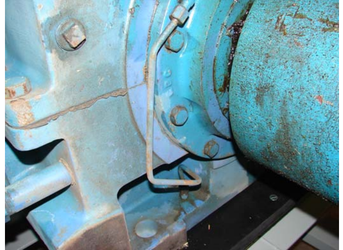
Figure 18. Low Speed Grease Supply Line
