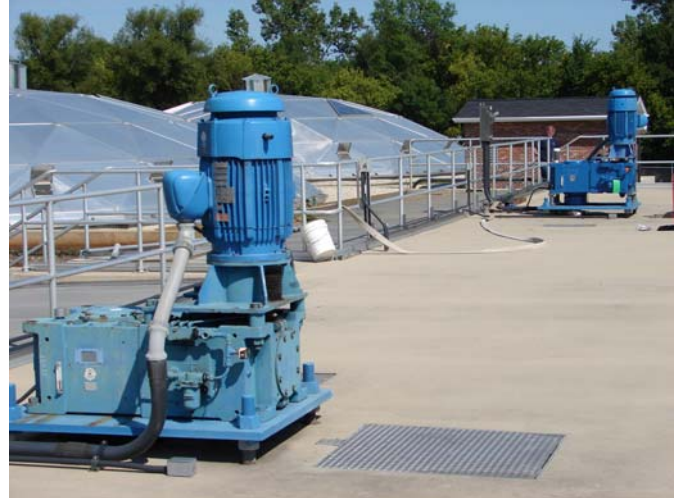
Figure 3. Aerator 1 (Original - Left), Aerator 2 (Replacement - Right)
