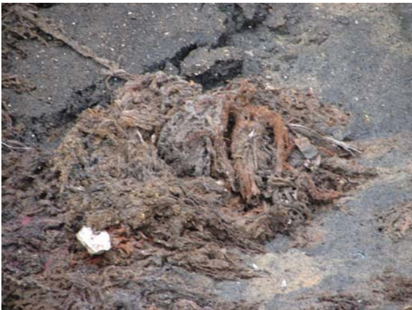
Figure 7. Detail of Fibrous Debris in Aerator 1 Basin
